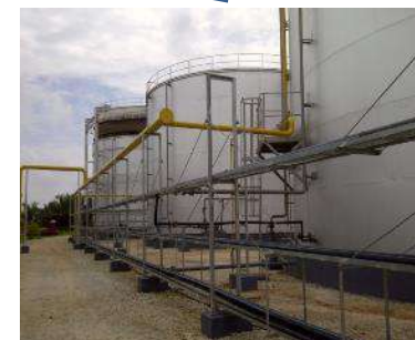
Tank Digesters : 51 units
